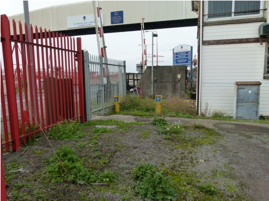
Photograph 26: St. Andrew's level crossing control cabinet
