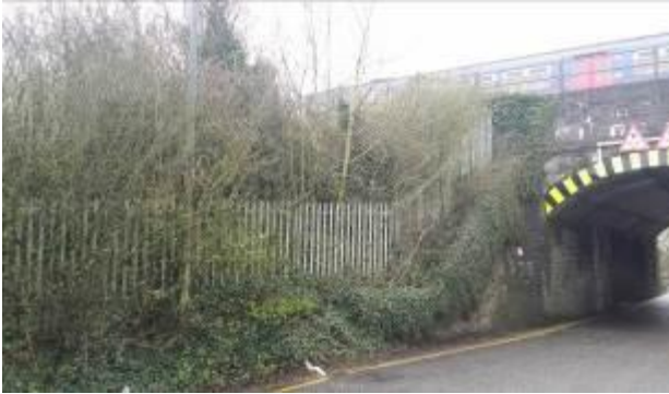
Vegetation to top of wing walls and parapets
