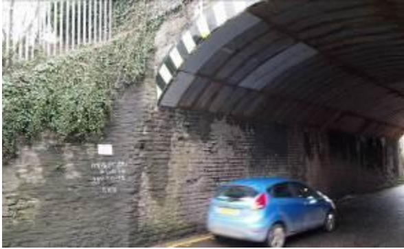
Wet staining, rust staining to sheeting, spalling and open joints
